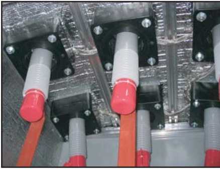
Interior of medium voltage compartment showing bushings with optional current transformers
